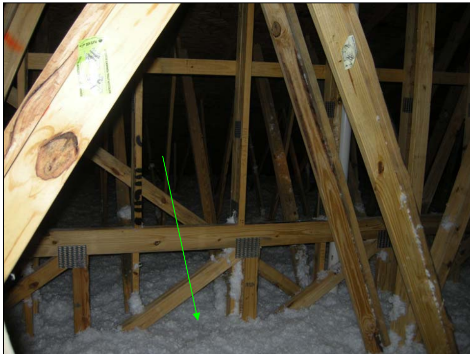
ATTIC – View of 'blown-in' thermal insulation - (Green Arrow) Three story, wood framed apartments – Texas
