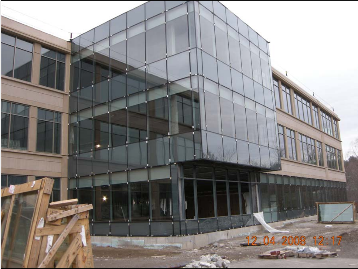
View of a Portion of the North Façade of New Headquarters Building Featuring Pre-cast & Curtainwall
