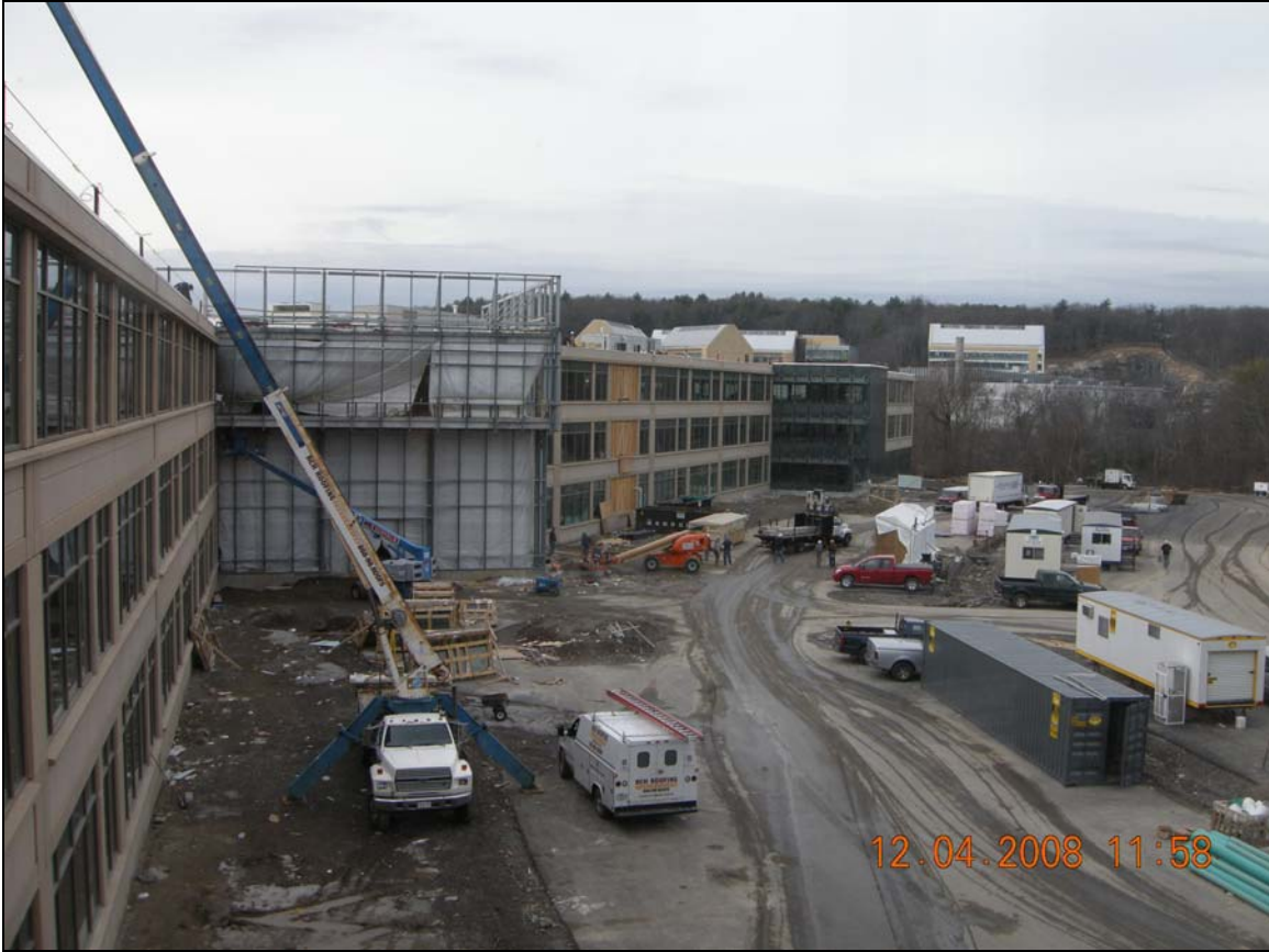
View of North Façade with Future Main Building Entry Atrium in Center
