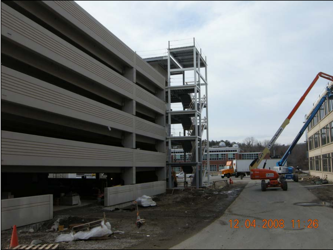
View of New Parking Garage in Progress (left) – Headquarters Building (right); Renovated VERIZON Building Beyond in Center
