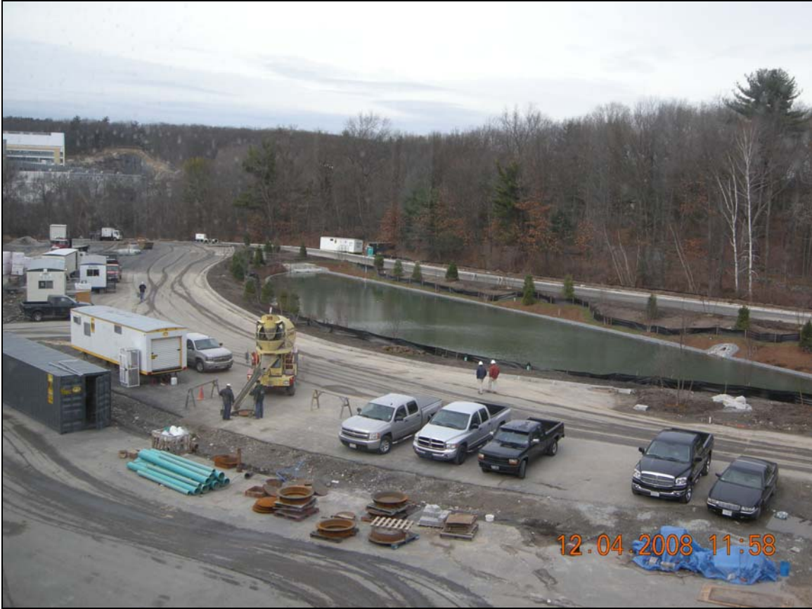
View of a Portion of Supporting Site Improvements Including Landscaped Storm Water Detention Pond
