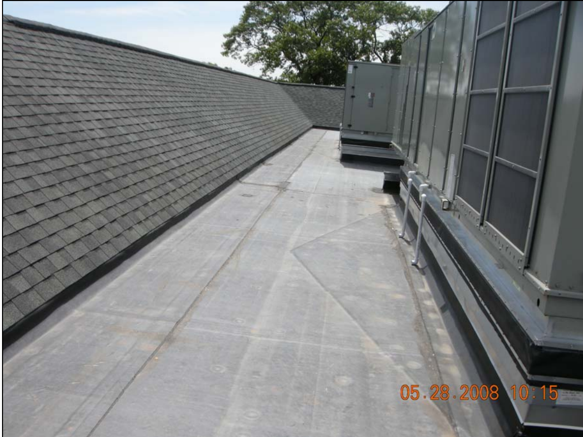
View of Roof Top Mechanical Equipment (HVAC) Behind Mansard Roof
